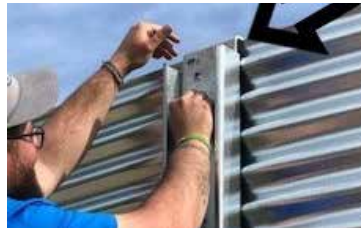
Figure 8 Installing Edge Beam on Top of Upright on 4th Ring of Panels
