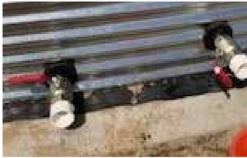
Figure 15 2" Inlet and 2" Outlet
